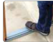
Low level door threshold
